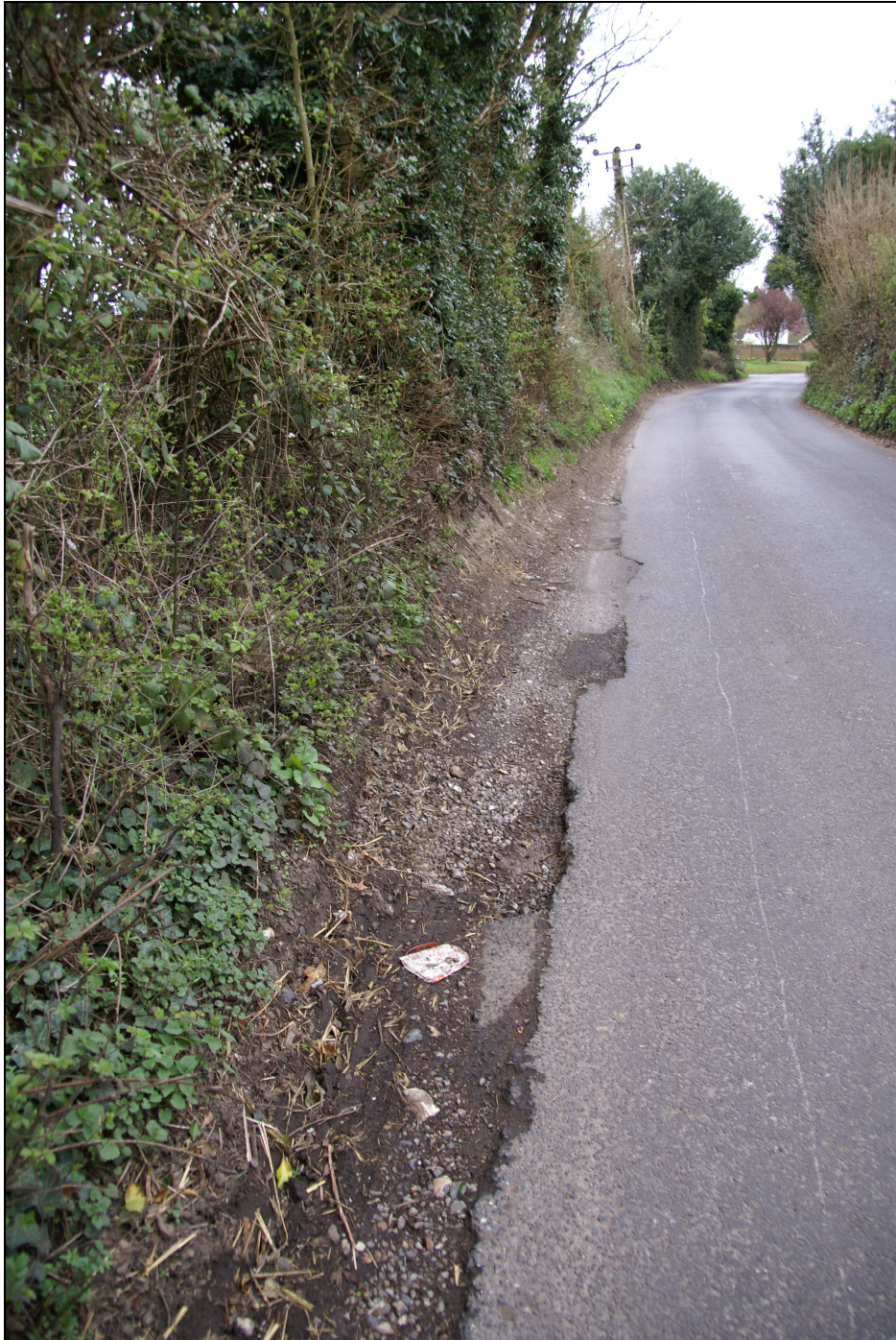
OVER-CUT HEDGEROW EXPOSING AND ERODING BANK AND CREATING POT HOLES
