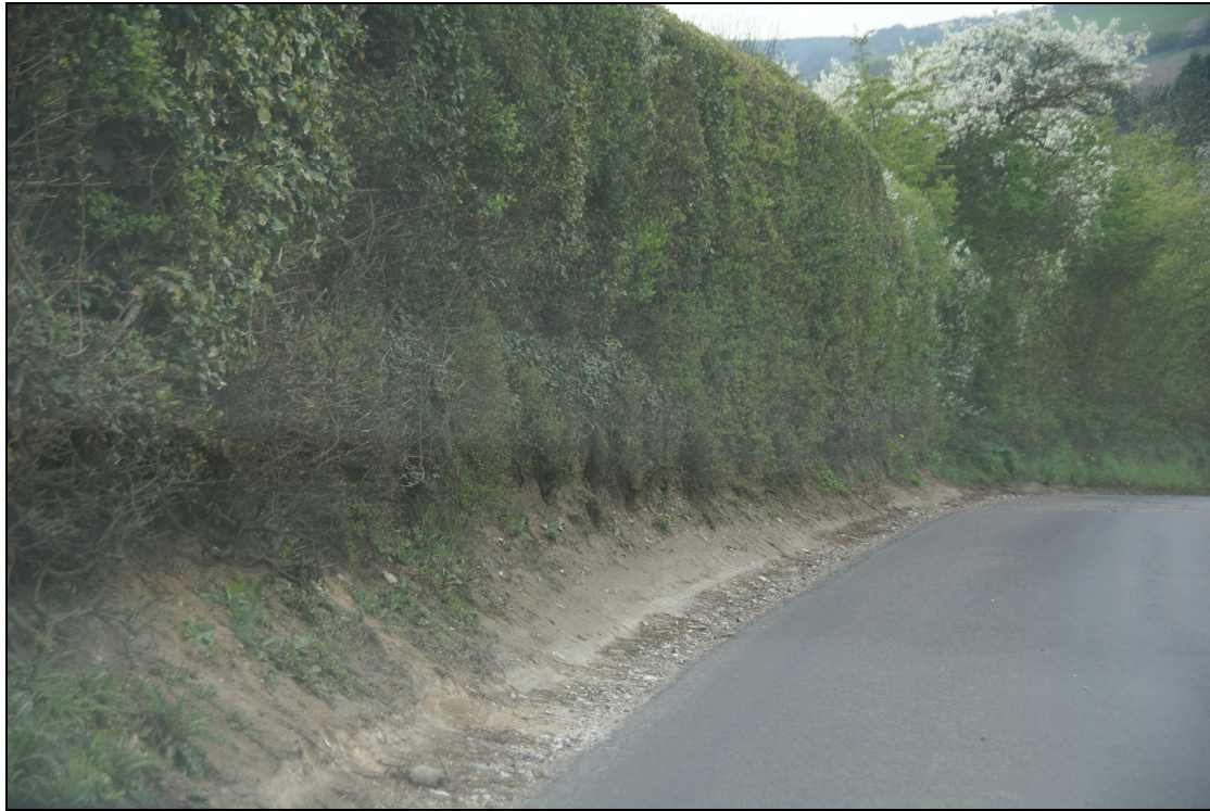
OVER-CUT HEDGEROW EXPOSING AND ERODING BANK AND CREATING POT HOLES
